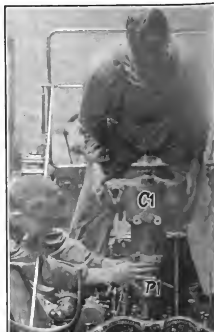
Fig. 2—Process of replacing cylinders, showing how two workmen guide cylinders over pistons without damaging the rings
